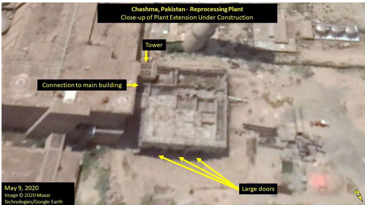
Image. The extension is near external completion in May 2020, with a roof structure covering roughly half of the extension.
