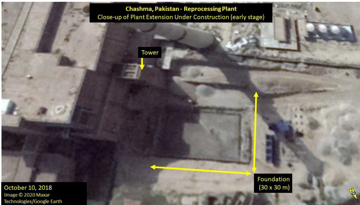
Image. By October 2018, a 30 x 30 m foundation for the extension below ground level is visible in Google Earth imagery.
