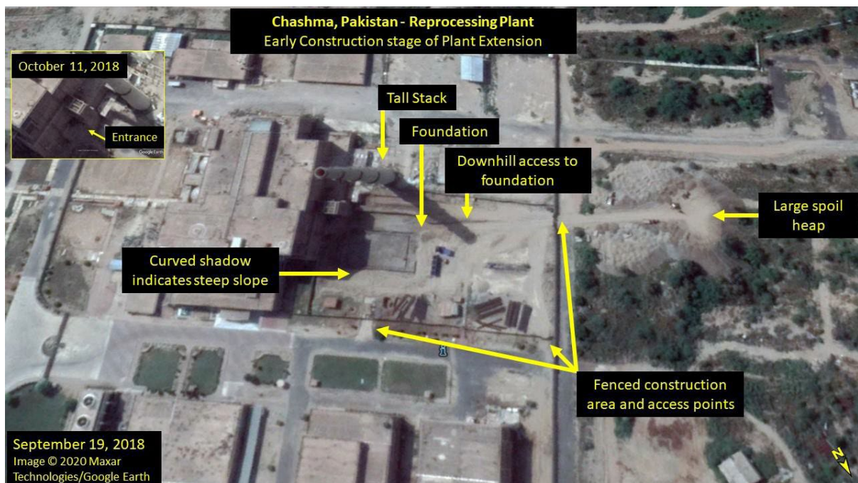
Image. The construction of the extension to the Plutonium Separation Facility at an early stage in September 2018.
