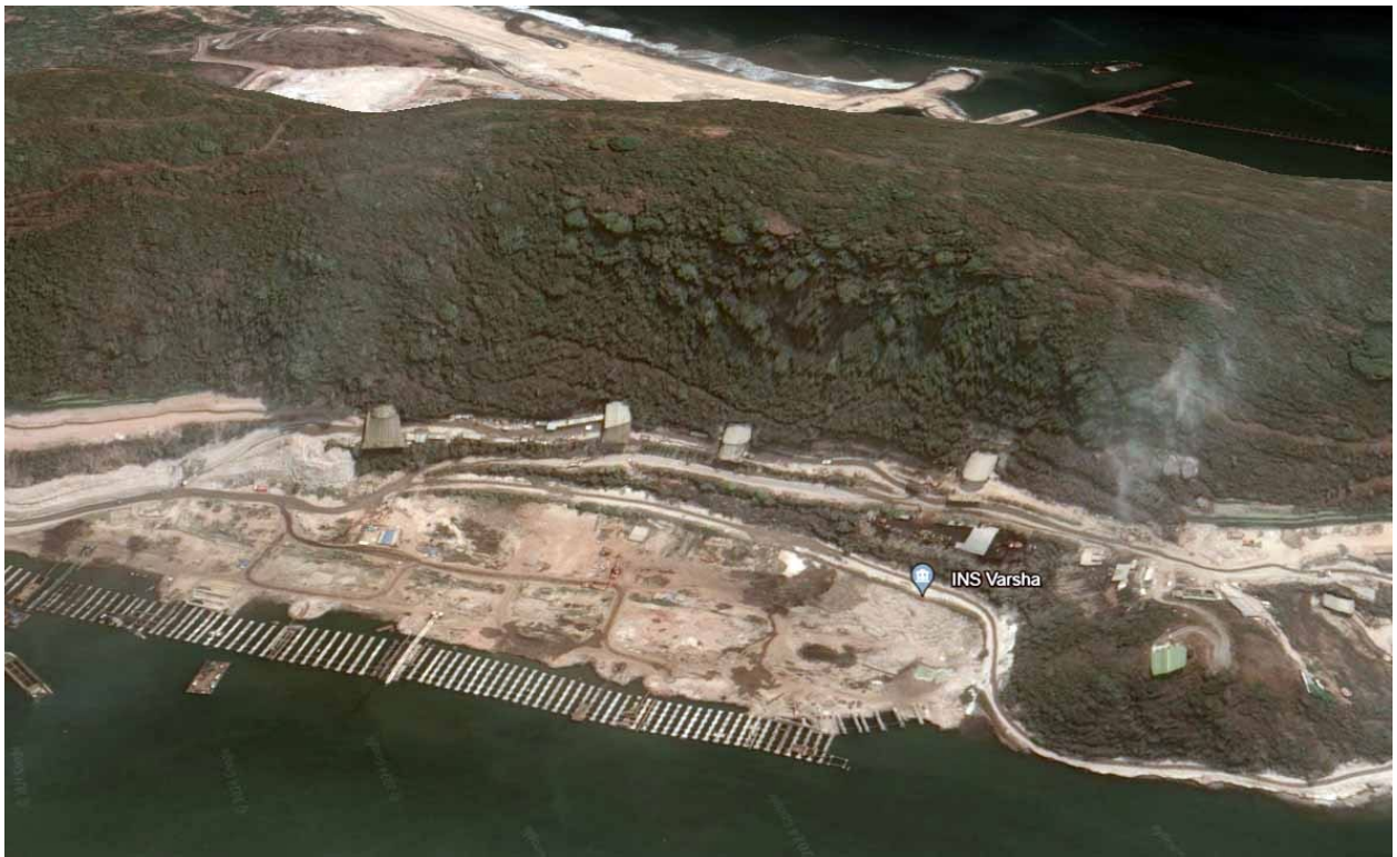
Image: The INS Varsha naval base under construction near Rambilli, India – copyright debuglies.com
